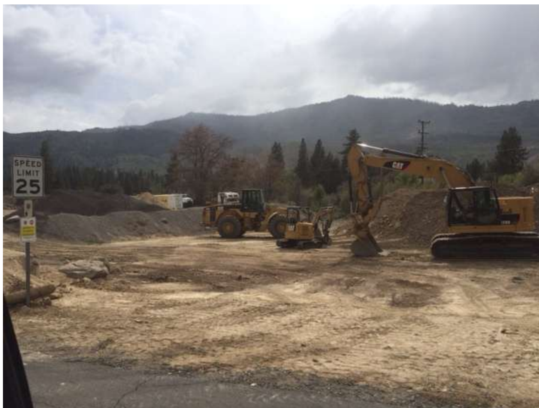
Figure 10. Construction at the 39 Ventures site, photo from May 13, 2015. Excavations including the one to the left foreground have the potential to expose contaminated material while new stockpiles can increase the expense of removal or other remedial actions.
