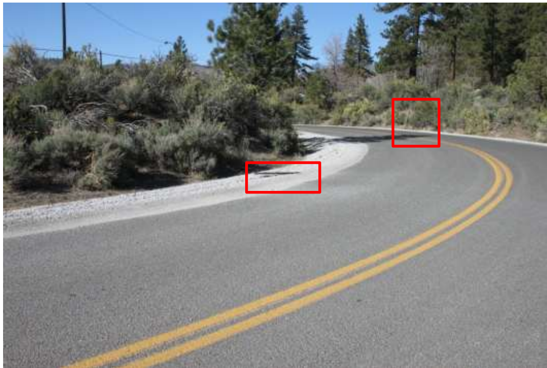
Figure 8. One of the curves between Interstate 80 access and the rail crossing on South Verdi Road. Note the damaged reflector posts in red rectangles where vehicles have been unable to navigate the relatively tight turns.
